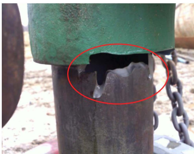
Figure 1—A fatigue crack at the wellhead-casing interface resulted in a blowout. The fatigue was vibration-induced.
